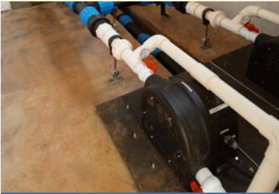
Turbines, Lwamba Hospital
