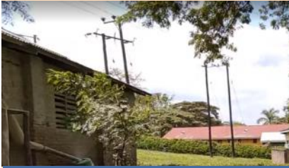
Kagando, existing electricity supply
