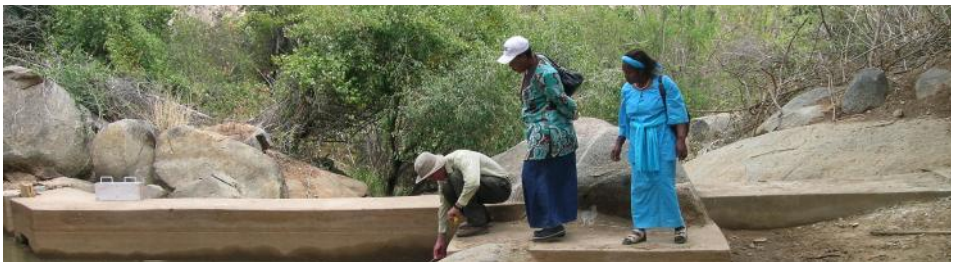
Tanzania, Pawaga. Intake for piped water supply, 2008-2011, serving 16,000 people in 8 villages on a 23km delivery pipeline at a cost of €1.2m. CED’s biggest project to date!
