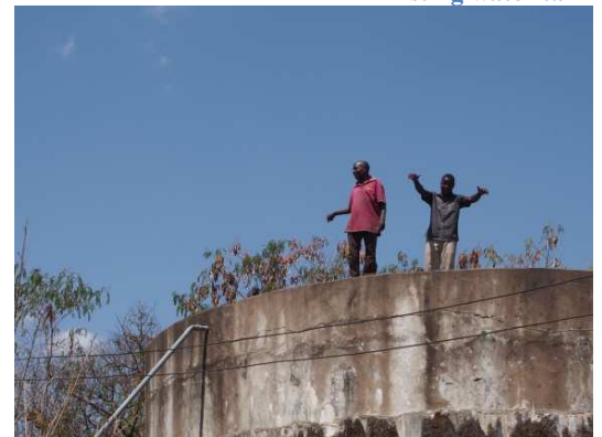
Water arrives at the tank
